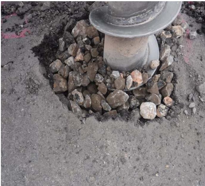
PHOTO NO. 31: General view of gravelly soils encountered in vertical boring B-8.
