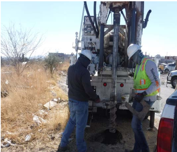
PHOTO NO. 47: General view of subsurface drilling operations at vertical boring B-13.
