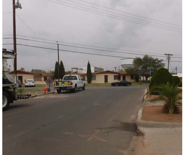
PHOTO NO. 16: General view of original pipeline route on Happer Street looking northeast.
