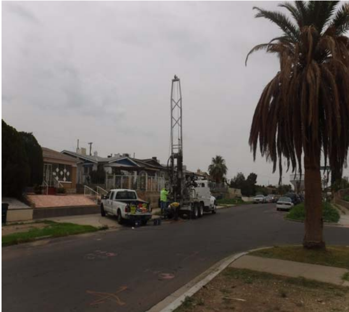
PHOTO NO. 23: General view of our subsurface soil drilling operations at vertical boring B-5.
