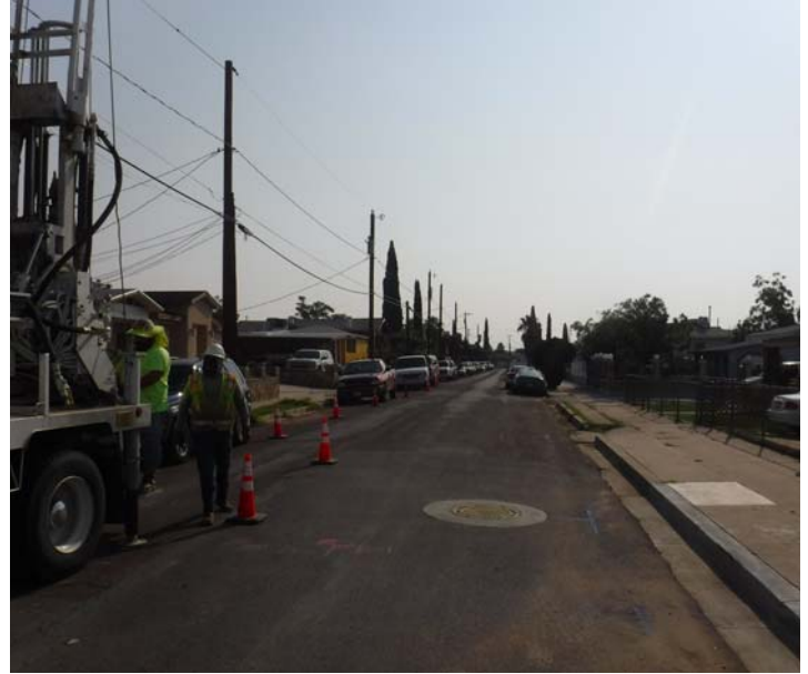
PHOTO NO. 2: General view of original pipeline route on Bishop Way looking northeast.
