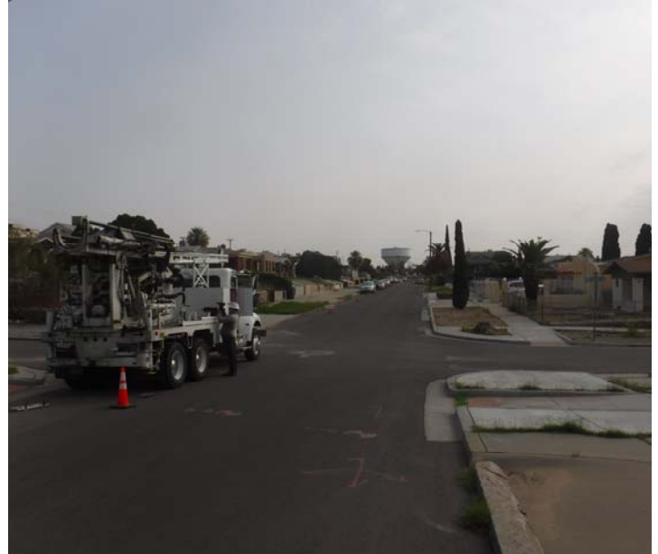
PHOTO NO. 8: General view of original pipeline route on Happer Street looking northeast.
