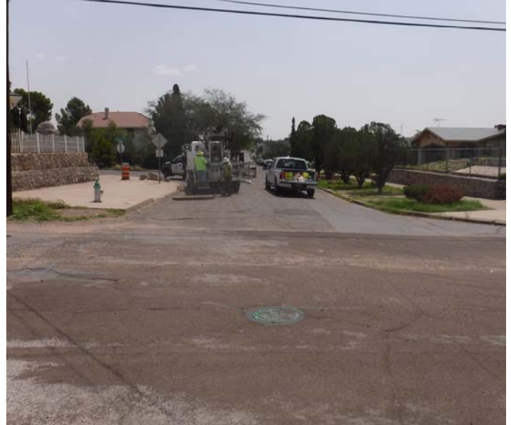
PHOTO NO. 6: General view of original pipeline route on Stevens Street looking east.
