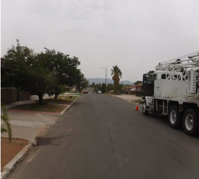
PHOTO NO. 15: General view of original pipeline route on Happer Street looking southwest.
