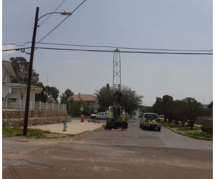
PHOTO NO. 22: General view of our subsurface soil drilling operations at vertical boring B-3.
