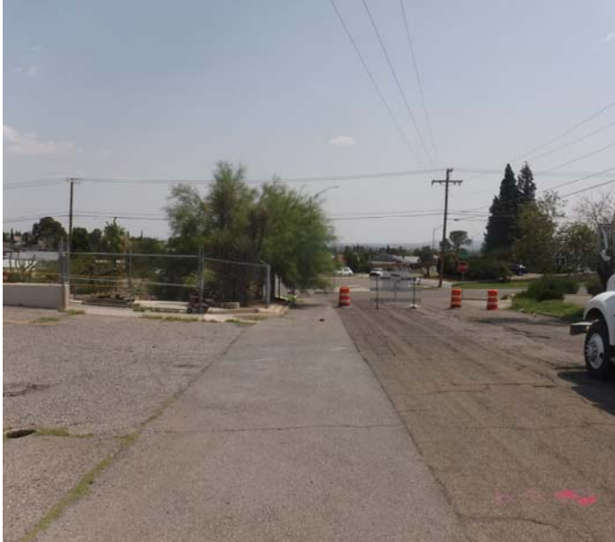
PHOTO NO. 17: General view of original pipeline route on Sparkman Street looking south.
