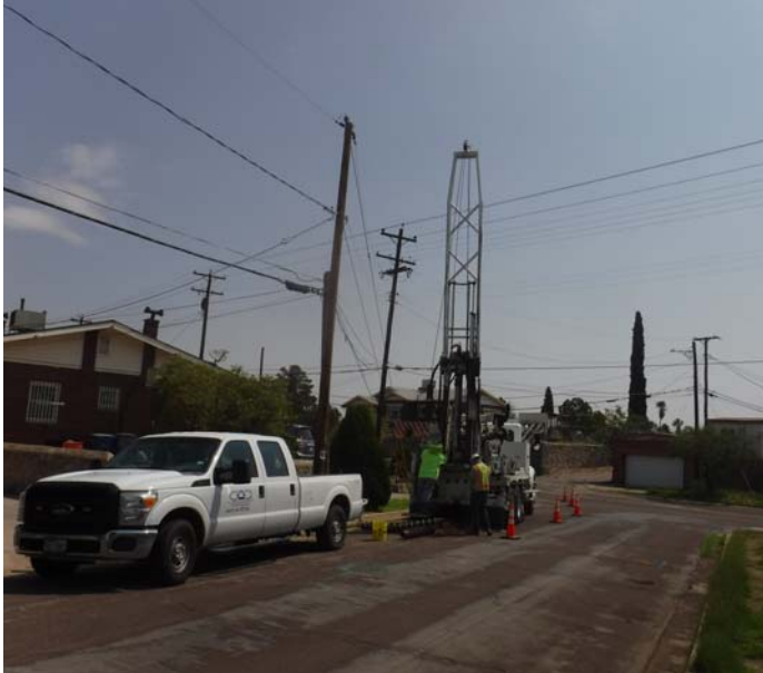
PHOTO NO. 21: General view of our subsurface soil drilling operations at vertical boring B-2.
