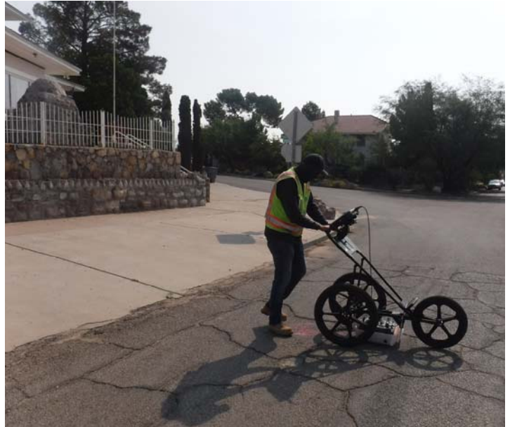
PHOTO NO. 34: General view of our ground penetrating radar operations on Cambridge Avenue.
