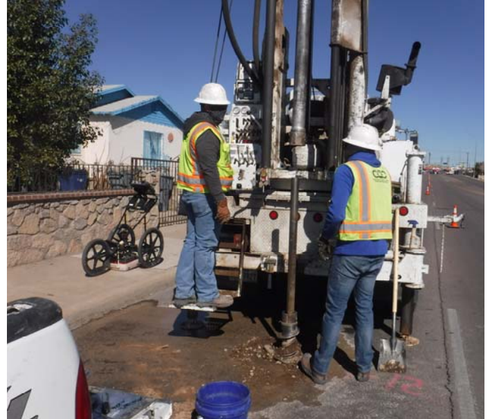
PHOTO NO. 46: General view of subsurface drilling operations at vertical boring B-12.
