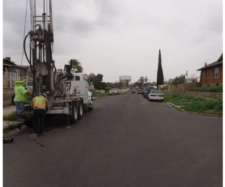
PHOTO NO. 10: General view of original pipeline route on Happer Street looking northeast.
