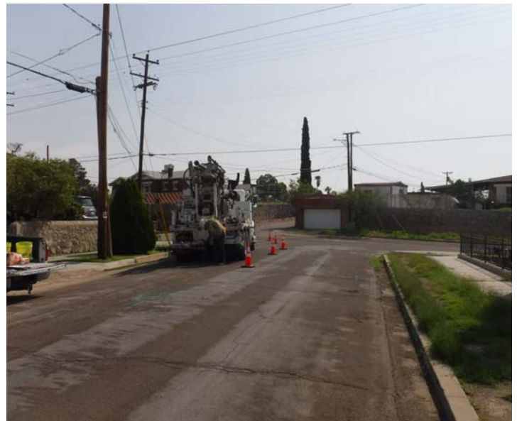
PHOTO NO. 4: General view of original pipeline route on Bishop Way looking northeast.
