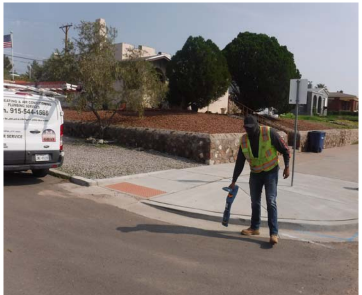
PHOTO NO. 36: General view of our utility locate operations on Happer Street.
