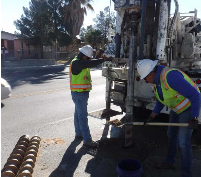
PHOTO NO. 45: General view of subsurface drilling operations at vertical boring B-11.
