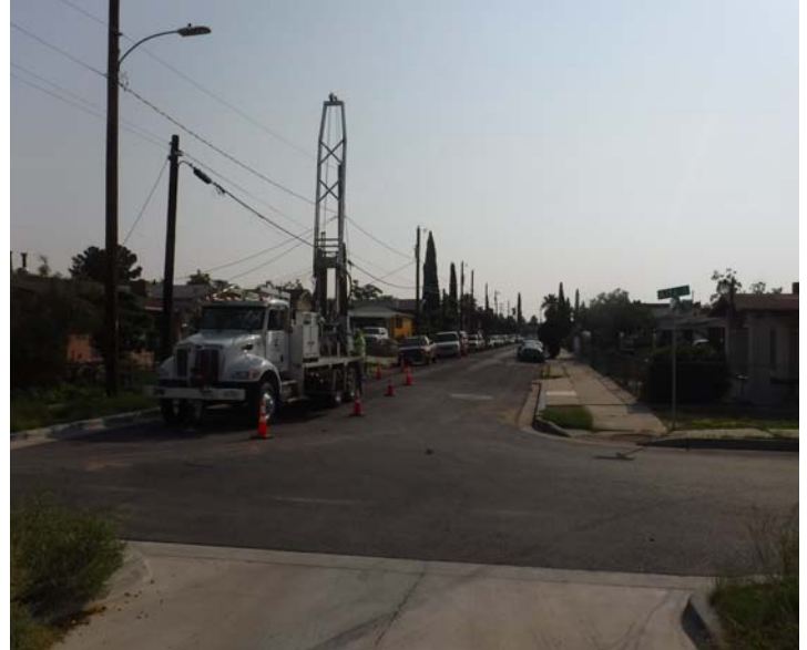
PHOTO NO. 20: General view of our subsurface soil drilling operations at vertical boring B-1.
